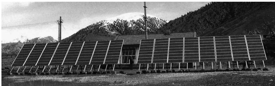
Fig. 15. A photograph of a stand-alone PV application.
